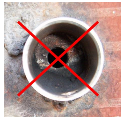
Figure 8 Wrong socket installation
