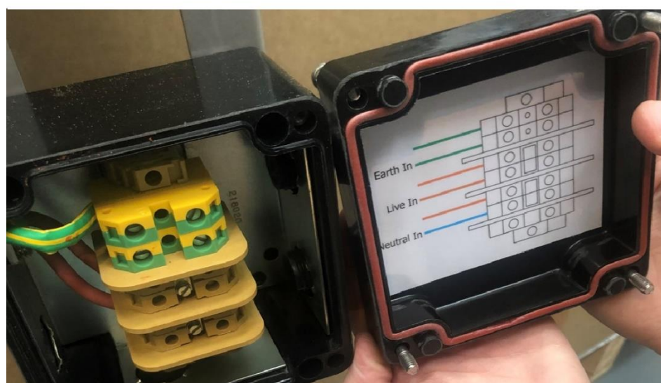
Figure M-2 The Junction Box of the In-situ Heater (Heater Tape Version)
